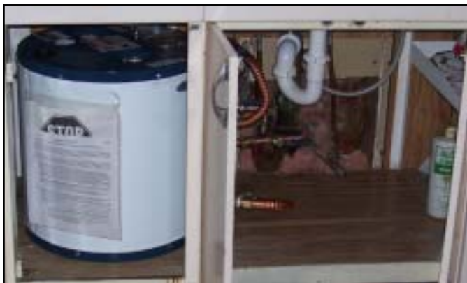
HOT WATER HEATER PHOTO, JOHN, W1ZYV
